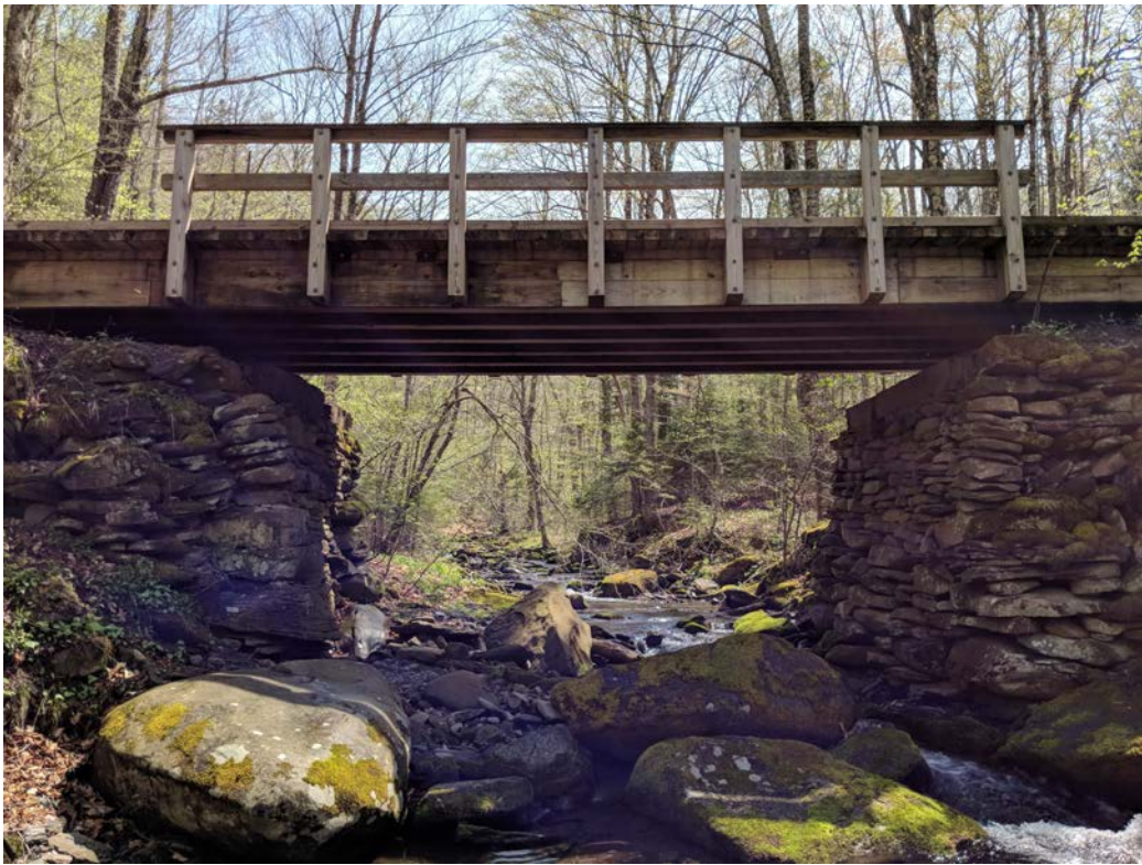
Bridge along the Spruceton trail. Photo by Stash Rusin, 2nd Vice President
